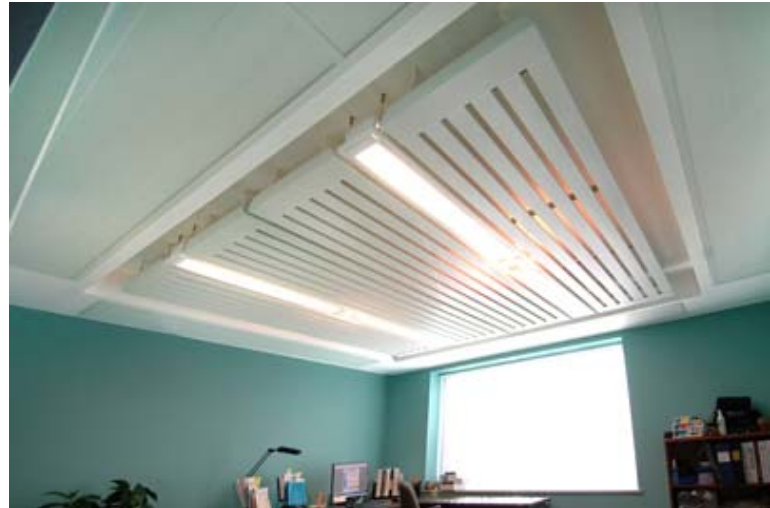
Figure 11.1.2. Radiant panel in an office h
